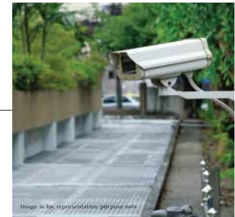
CCTV surveillance in Common Areas
